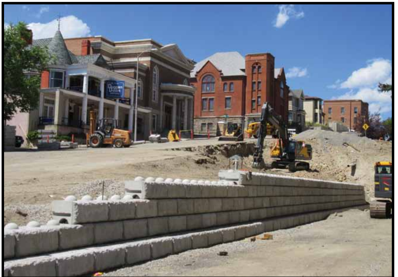
Work is progressing to replace a retaining wall on the west side of the Courthouse and to realign Montana Street. Photo by Robin Jordan
