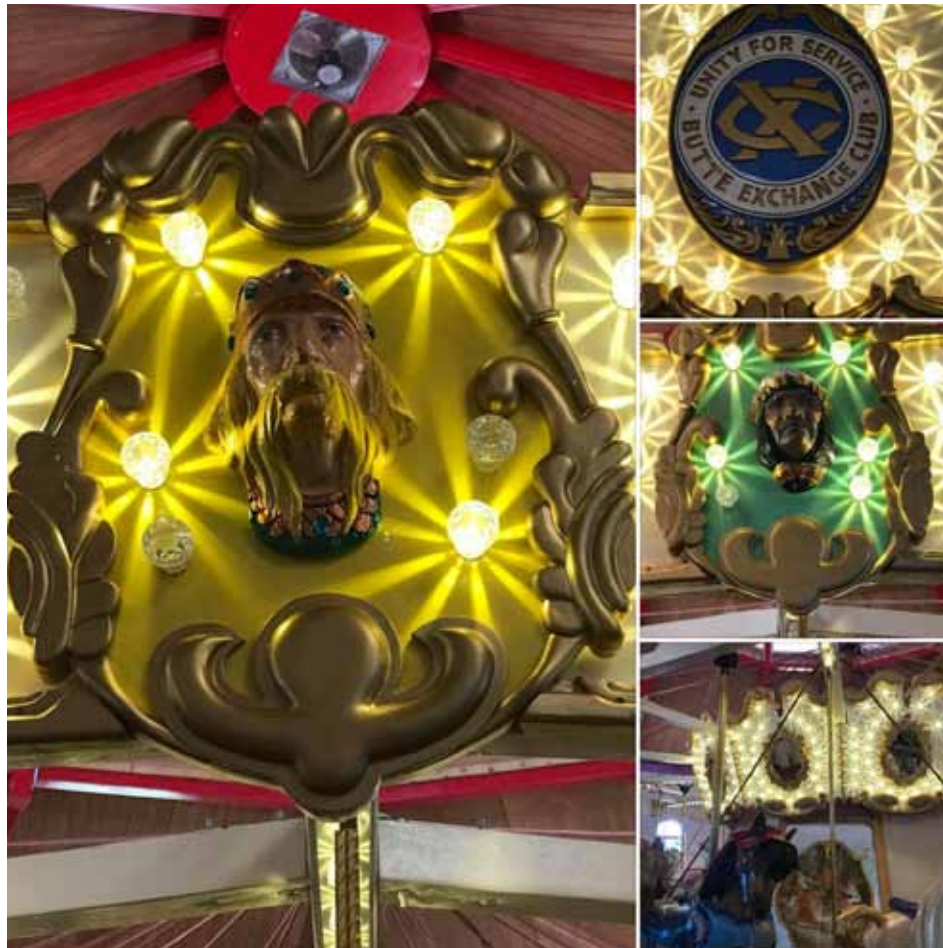
Here are photos showing electrical progress yesterday. Our electrical volunteers often can only work weekends and nights.
